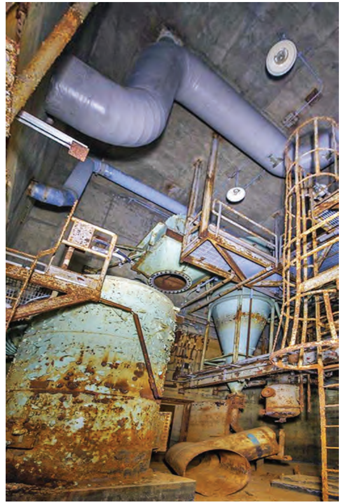
The combustion air room of prime mover module 4. Photo Chris Howells
